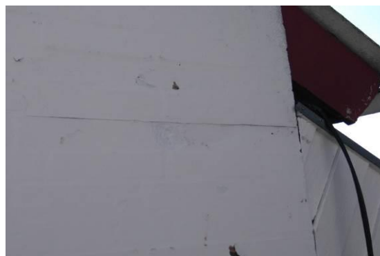
Revne i gavl
