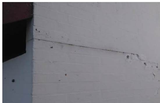
Revne i gavl
